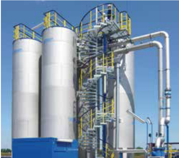
Source: DynaSand filter from Nordic Water/Water
